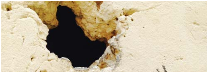
BEFORE —The Benton Building's limestone was heavily coated with atmospheric staining and significantly deteriorated.
