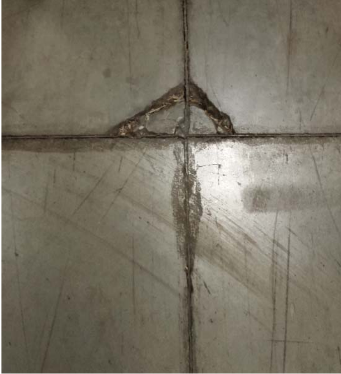
BEFORE - Geological issues below the slab and heavy forklift traffic cause deflection and excessive floor joint damage.
