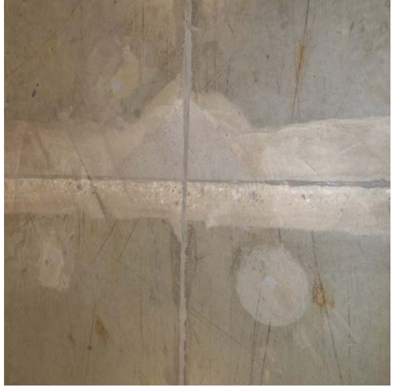
AFTER - With multiple types of floor joint repair methods, floor slab stabilization techniques and high density foam injection.
