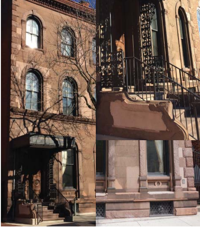
BEFORE —Weathering, age induced decline, pollutants, and acid rain has accelerated the breakdown of the veneer materials.
